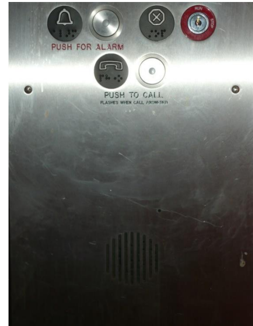
Elevator Emergency Phone Box
