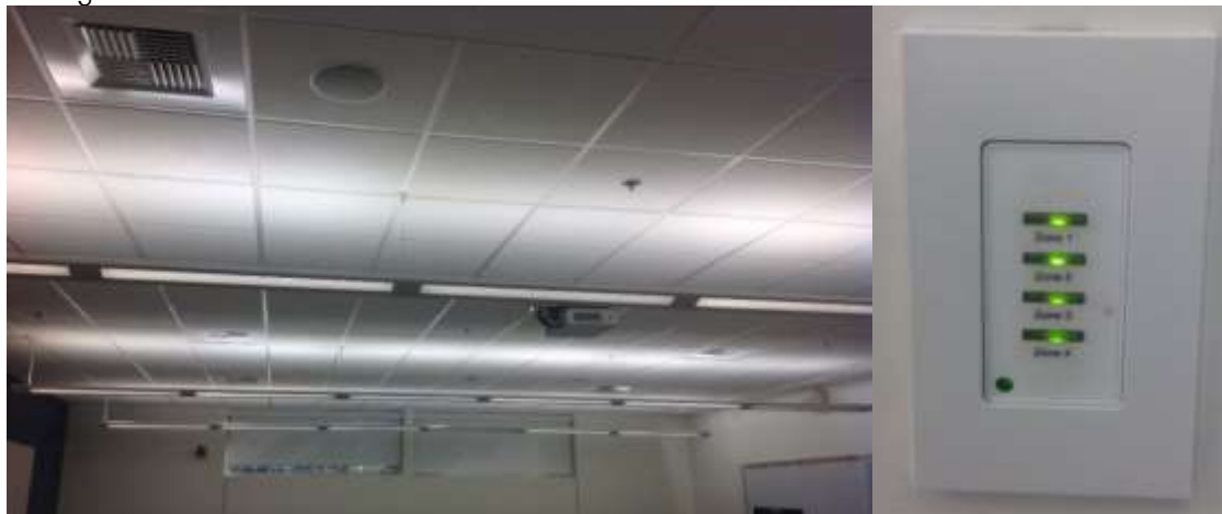
Figure 49: LED Lighting and Controls as Installed in the Nursing Building
