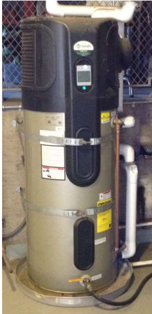
Figure 46: Air-to-Water Heat Pump, Installed in LA1
