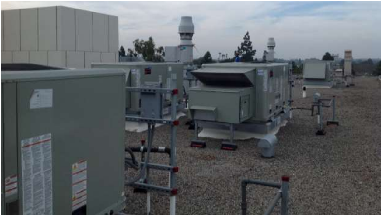
Figure 36: Modern RTUs Recently Installed on Roof of Psychology Building
