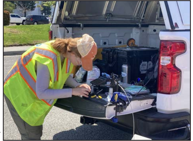
FUSION OF FIBER OPTIC CABLE AT PM-07 MONITORING WELL IN TORRANCE, CA.
