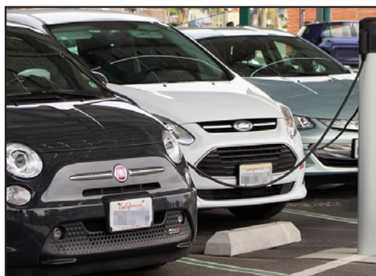
Additional EV charging spaces
