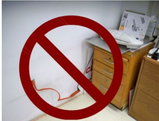
Not OK: extension cord
